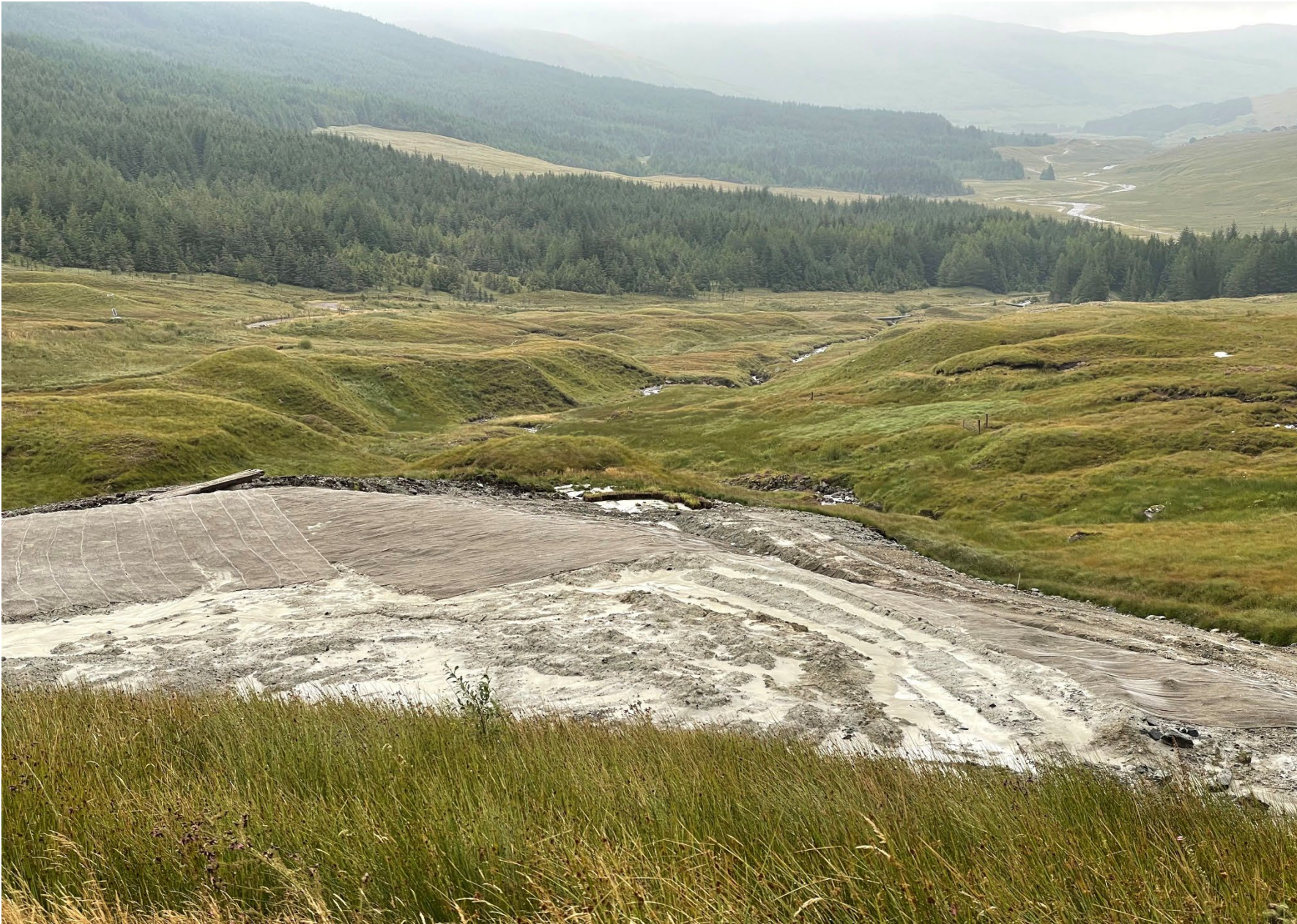
Stack 2, Geojute secured across the majority of the Stack with a small opening retained to receive silt from pond clearance works
