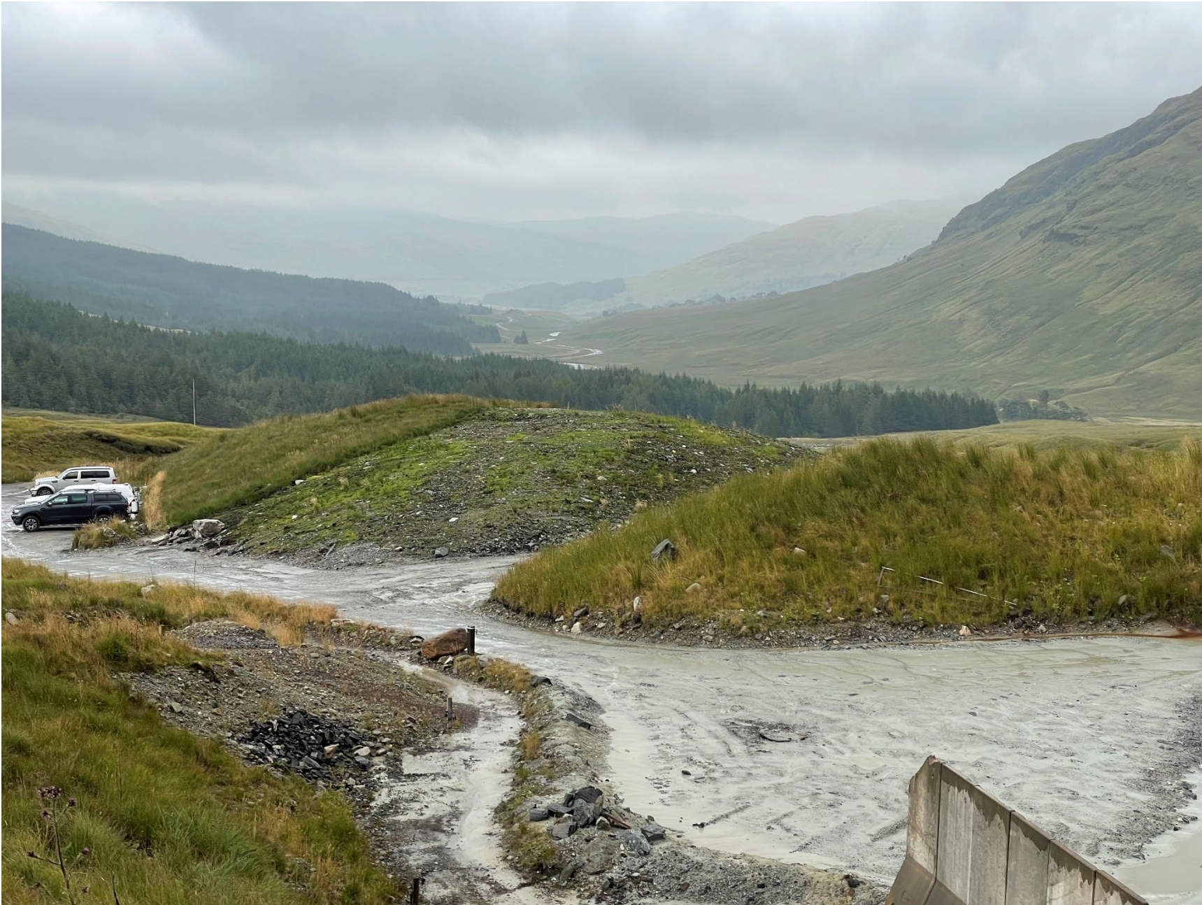
Stack 1, Seeded areas are establishing and turfed areas have developed thick growth. Platform bund (foreground) well establish thick growth
