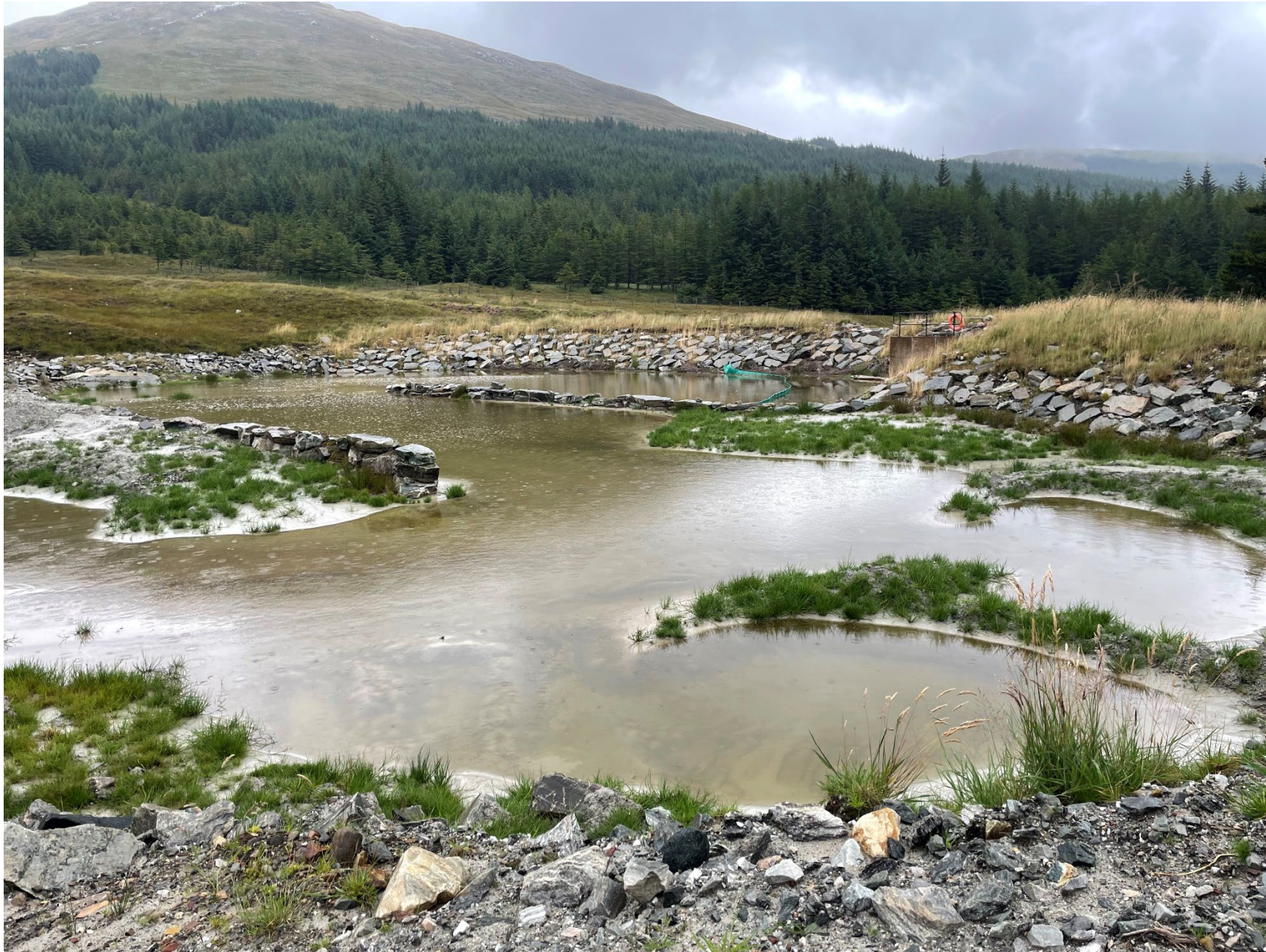
TMF Settlement Pond, Below capacity with sediment boom retained, further clearance planned early October
